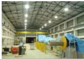
Workshop with induction lighting in India
