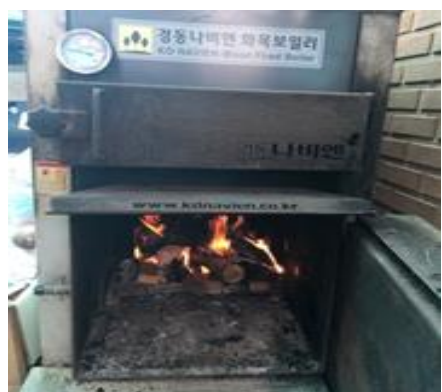
The wood-fired boiler
